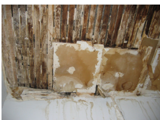
Mr. C’s ceiling caving in from extremely leaky roof
